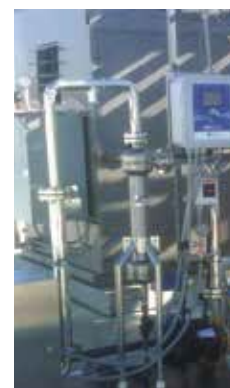
ILS used to remove solids from water supply system for a large grocery store.
